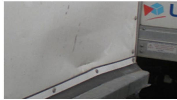
🔧 Side and rear doors: Significant deformation: Repair time > 1 h within economic repair; closure not sealed
